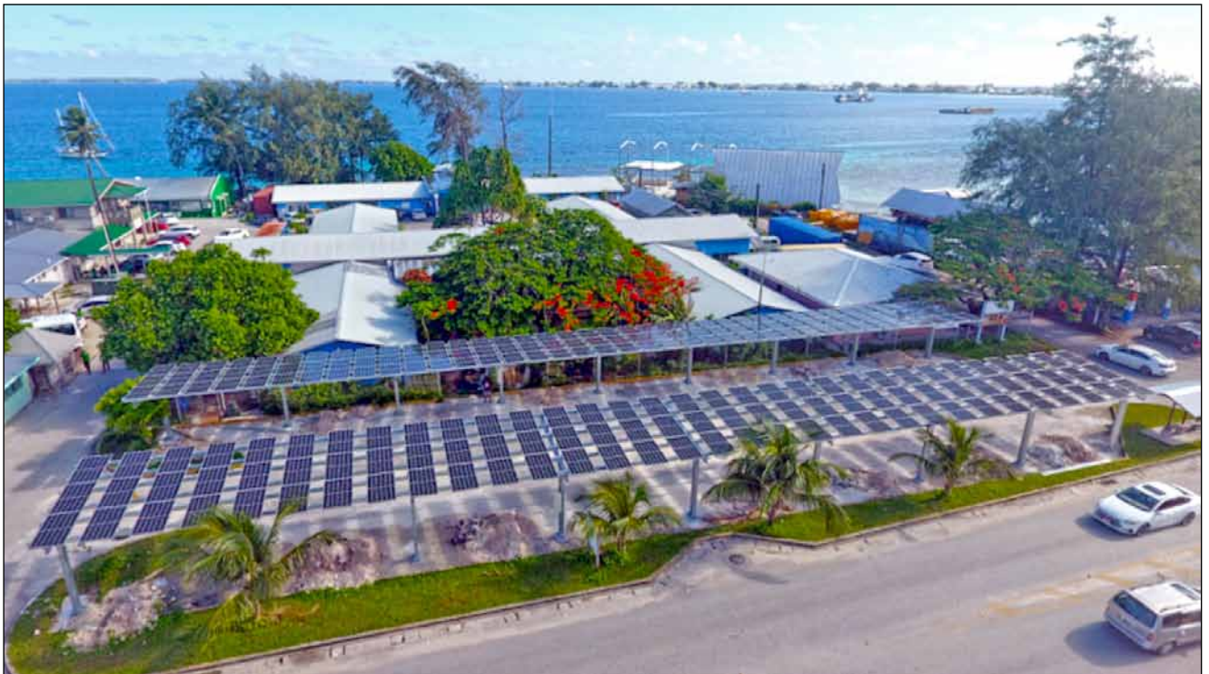
Figure 1: PSS Solar Parking lot. PC: Green Energy Solution
